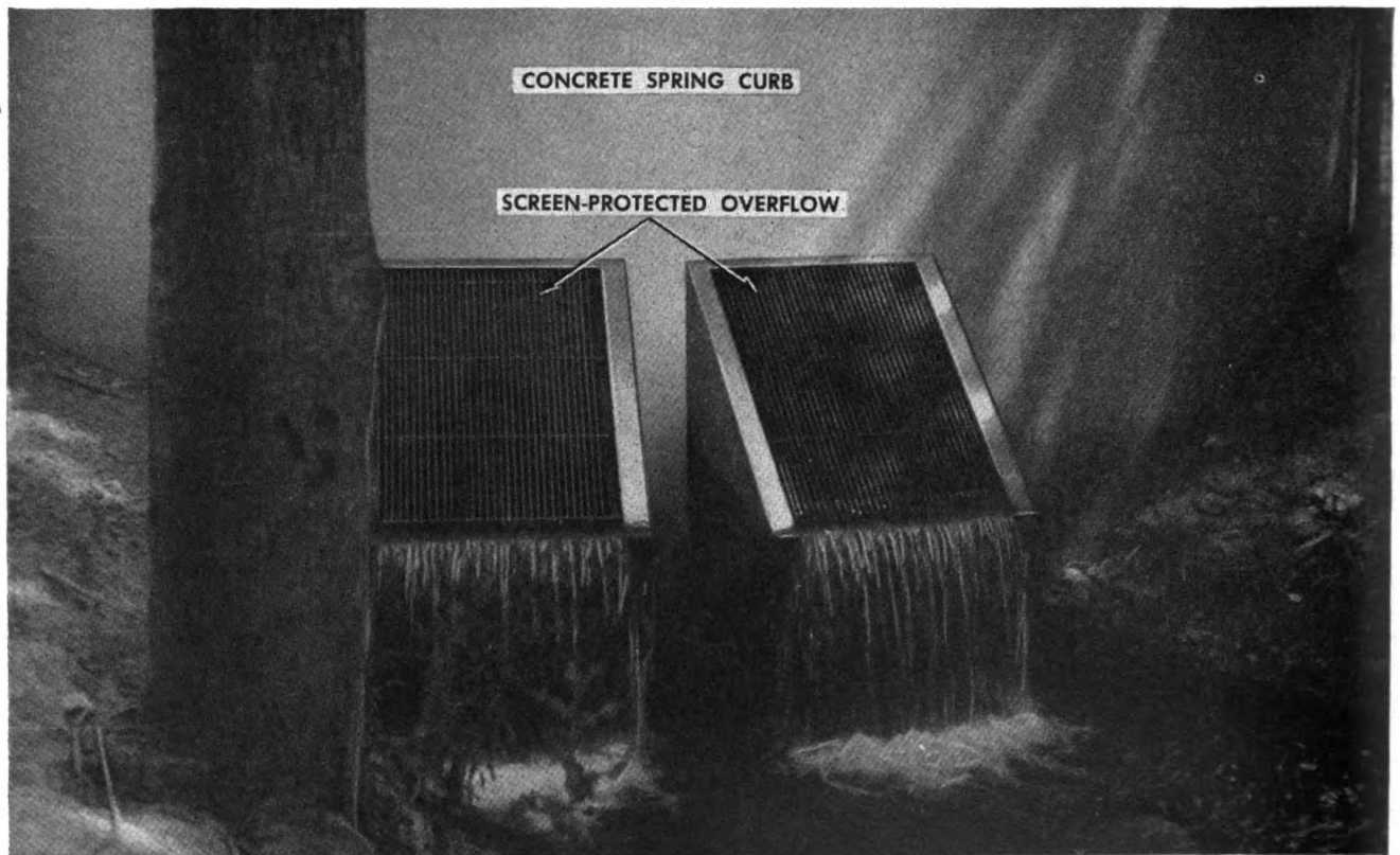
Figure 26. Spring protected from contamination by concrete curb and screening on overflow.
